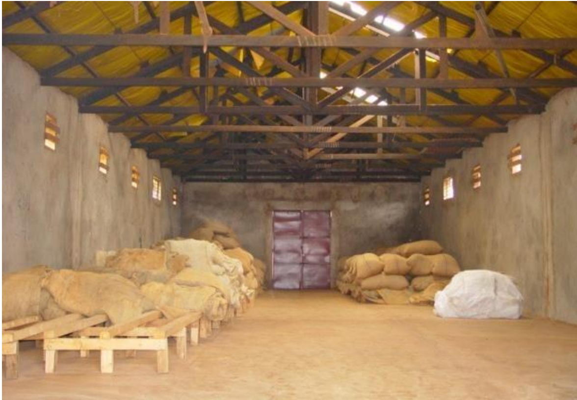
Figure 4.1: Properly designed coffee store with insulated roof and fitted with wooden pallets
