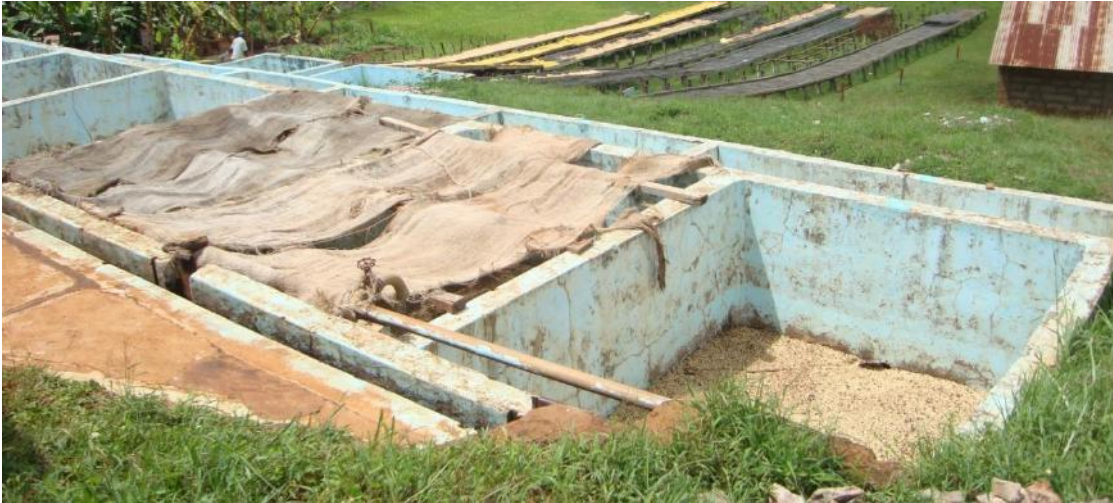
Figure 8.6: Poorly maintained fermentation tanks with no roof
